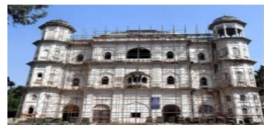
The restoration work of Butler Palace in Lucknow is under way and it is expected to complete in next six months. SANDEEP SAXENA
