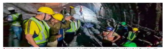
A way out: Rescue work under way at the tunnel in Uttarakhand district of Uttarakhand on Tuesday. PTI
