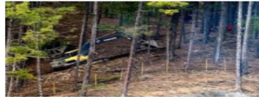
An earthmover deployed on top of the tunnel to pursue vertical drilling, in Uttarakashi on Saturday. SHASHI SHEKHAR KASHYAP
