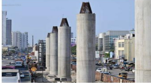
In progress: Construction work of the Chennai Metro Rail's Phase 2 at OMR, Chennai. SBANATH M
