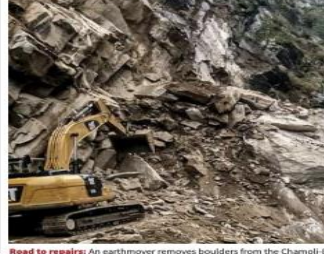
Road to repairs: An earthmover removes boulders from the Chamoli-Badrinath National Highway following a landslide on Sunday, Aug 4
