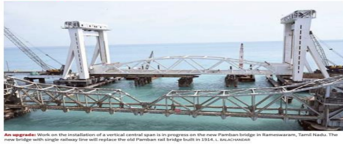
An upgrade: Work on the installation of a vertical cantilever span is in progress on the new Pamban bridge in Rameswaram, Tamil Nadu. The new bridge with single railway line will replace the old Pamban rail bridge built in 1914. L. BALACHANDAR
