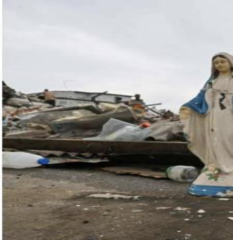
A statue of the Virgin Mary amidst the rubble of homes demolished at Adjame village in Côte d'Ivoire. Clashes broke out between the police and hundreds of residents of Adjidan on Thursday morning during a demolition and eviction drive. AFP
