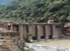
A section of the Teesta power plant damaged by a glacial lake outburst flood in October 2023.
