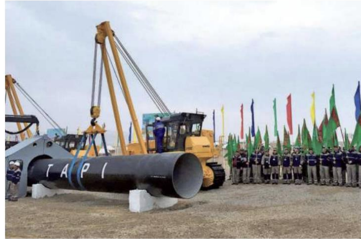
Slow progress: Work on the pipeline has been delayed by security issues in Afghanistan. FILE PHOTO
