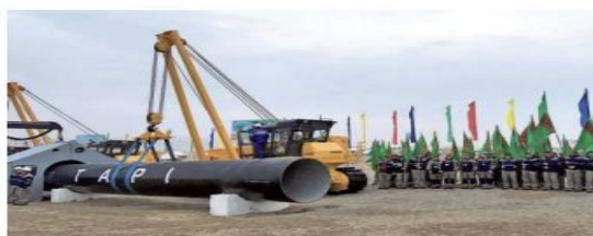
Slow progress: Work on the pipeline has been delayed by security issues in Afghanistan. FILE PHOTO
