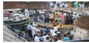
Fatal fall: Rescue operation under way after a house collapsed in Meerut on Saturday.
