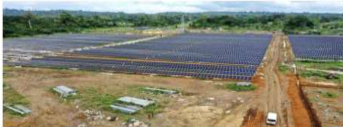
See friendly initiatives: This aerial view shows photovoltaic panels at Plain Agri solar plant in Foshing, on the outskirts of Gaborone. The plant spans some 100 hectares and was developed by Dubai-based SDEH. The project aims at producing 120 MW of power to supply electricity to thousands of households in Gaborone upon its completion, becoming the largest solar facility in Central Africa equipped with a battery Energy Storage System (BESS). AFP
