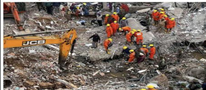
Ground zero: Rescue operations continued on Sunday after a multi-storey building collapsed at Sobhana village in Mohali district of Punjab on Saturday evening. Two people were killed in the accident. » PAGE 6
