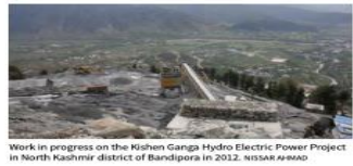
Work in progress on the Rishan Ganga Hydro Electric Power Project in North Kashmir district of Bandipora in 2012. NISAR/ANAD
