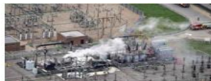
Energy crisis: Smoke billows from a substation in Heathrow Airport amid efforts to douse the fire that broke out on Friday. AFP
