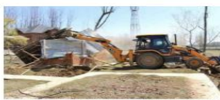
The police say they demolished an illegal structure on property linked to a Pakistan-based LeT handler. @ANWARPOOL/PTI
