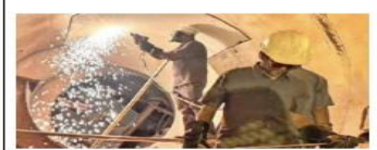
Tough task: Rescue operation underway to trace the workers trapped inside the partially collapsed SLBC tunnel on Saturday. PTI
