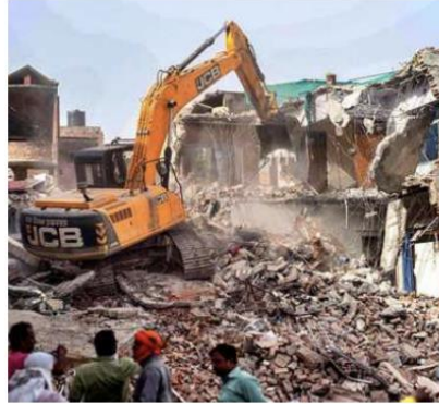
Bulldozer being used to demolish an ‘illegally built’ house in Prayagraj of Uttar Pradesh. FILE PHOTO
