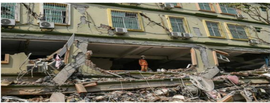
Collapsed dreams: A rescue worker looks out over the rubble as teams attempt to free trapped residents at the destroyed condominium in Mandalay on Saturday. AFP
